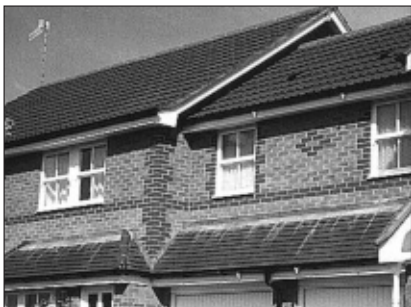
Roof tiles spoiled by run-off staining.
